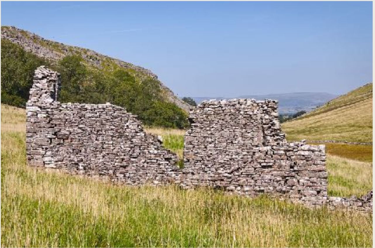
South elevation, with no apparent doorways (top); North elevation with remains of cart entry (bottom).
