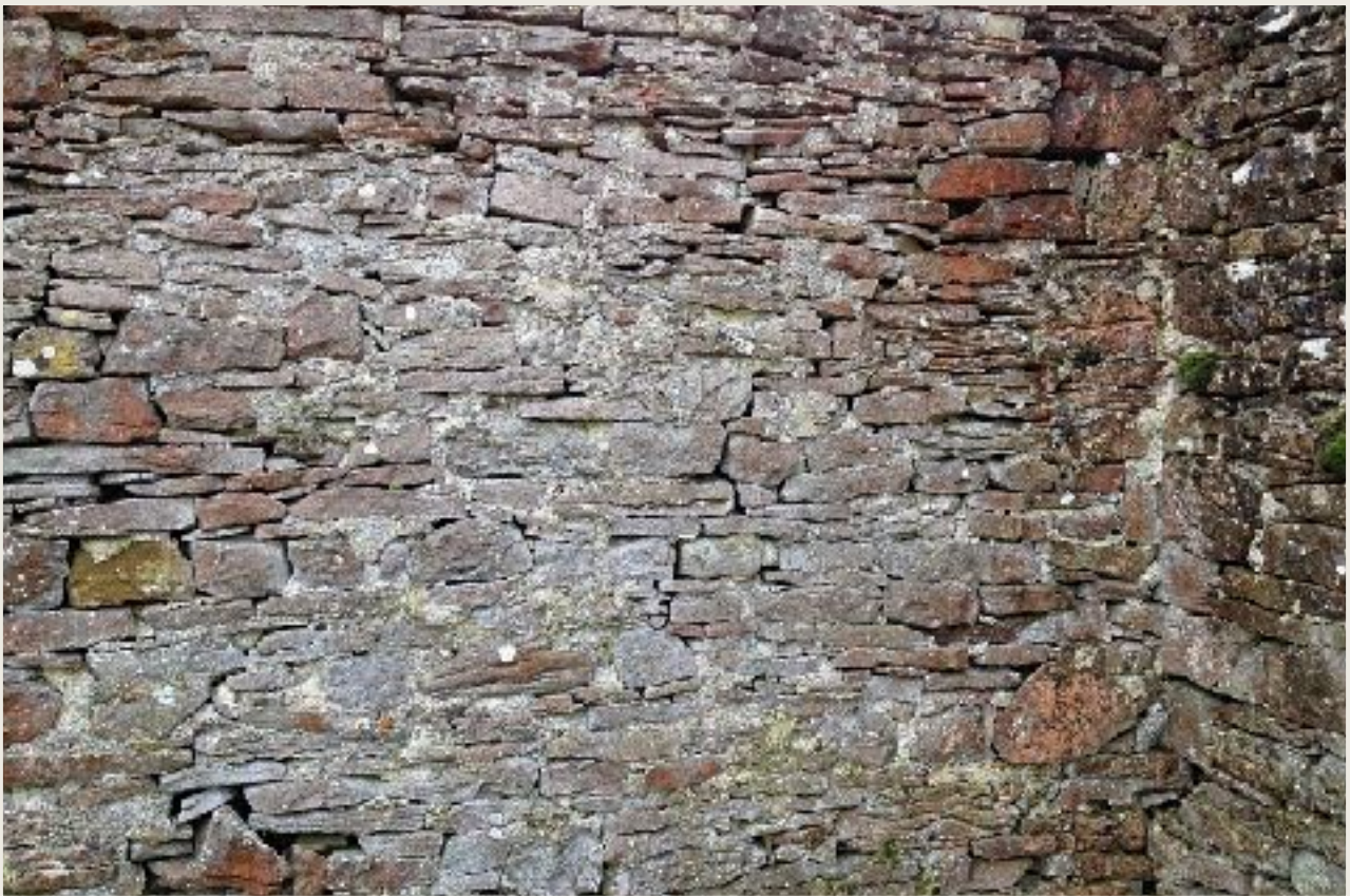
View of south elevation interior showing well mortared wall brought flush or rendered with a harl-like finish.
